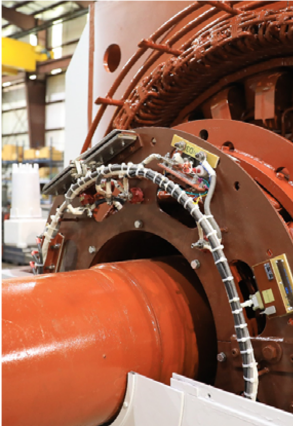
The modified exciter assembly was ready within 24 hours of the request for support from the customer
